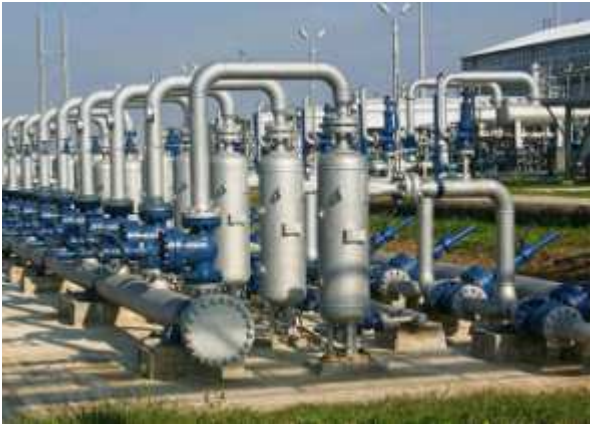
Fig. 35. Through the pipes shall be transported today all sorts of liquid chemical
