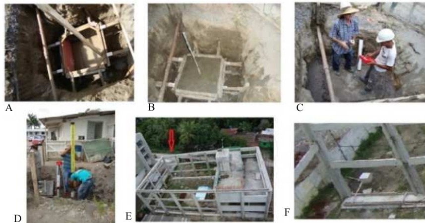
Fig. 2: Level References of the LITPEG work. A. Construction of RN LITPEG01; B. Concrete of the base and fixation of the metal rod; C. Fixation of BM; D. RN LITPEG01 and support of the rod sight; E. and F. Location of RN LITPEG02
