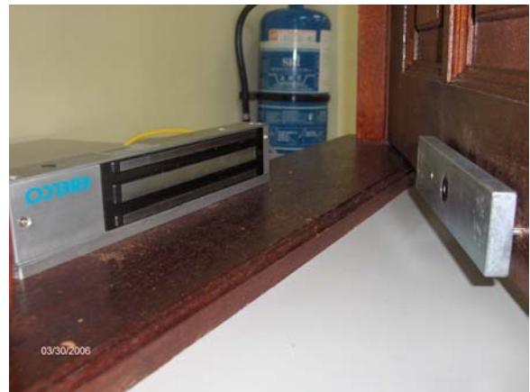
Fig. 2: Door with electromagnetic lock
